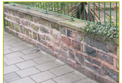
Figure 35: Examples of inappropriate pointing: Repointing of a sandstone wall where mortar joints appear over-dominant and strap or ribbon pointing
